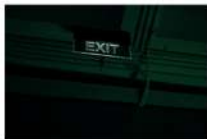
Detail shot of EXIT sign, illuminated in green.
